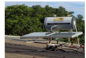
Our new solar water heater
